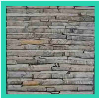
Broken Stacking Stone
